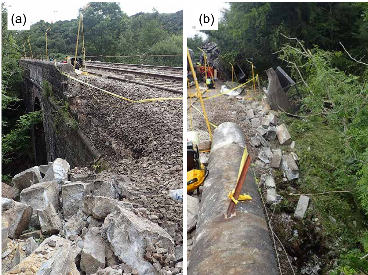
Figure F.8: Up-side parapet damage (a) looking south and (b) looking north
