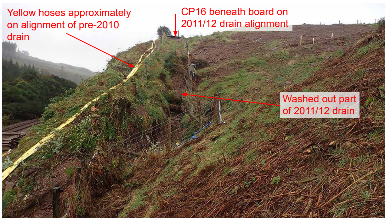
Figure G.2: View from near CP18 towards CP16 showing alignment of the pre-2010 crest drain and the 2011/12 drain after post-accident vegetation clearance
