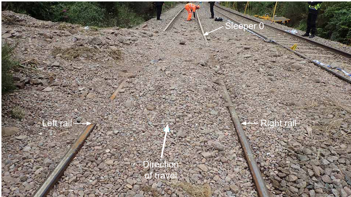
Figure 22: Washout debris covering the track and point of derailment at sleeper 0. Grooves cut by the wheels of train 1T08 through the debris are visible
