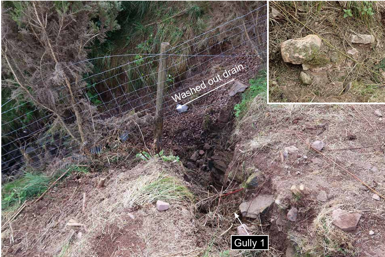
Figure 38: Gully 1 erosion at junction with 2011/12 drain (ORR/Coffey). Inset shows organic growth in base of gully 1 just outside main picture
