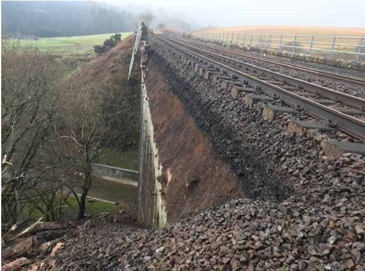
Figure M.2: Up line on bridge 328 looking south on 15 January 2021 (Network Rail)
