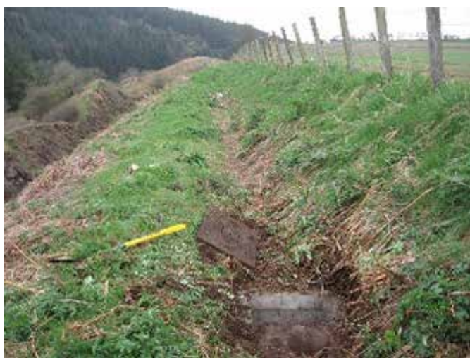
Figure G.1: Pre-2010 crest drain catchpit between CP10 and CP16 showing drain close to the cutting crest in 2010 (Carillion)
