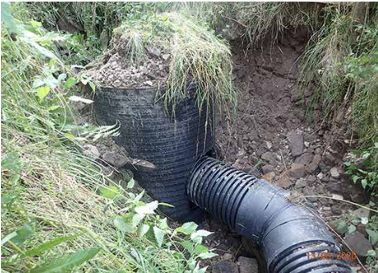
Figure 39: CP18 viewed from downslope on 13 August 2020 with the end of gully 2 visible at the upper right of the image
