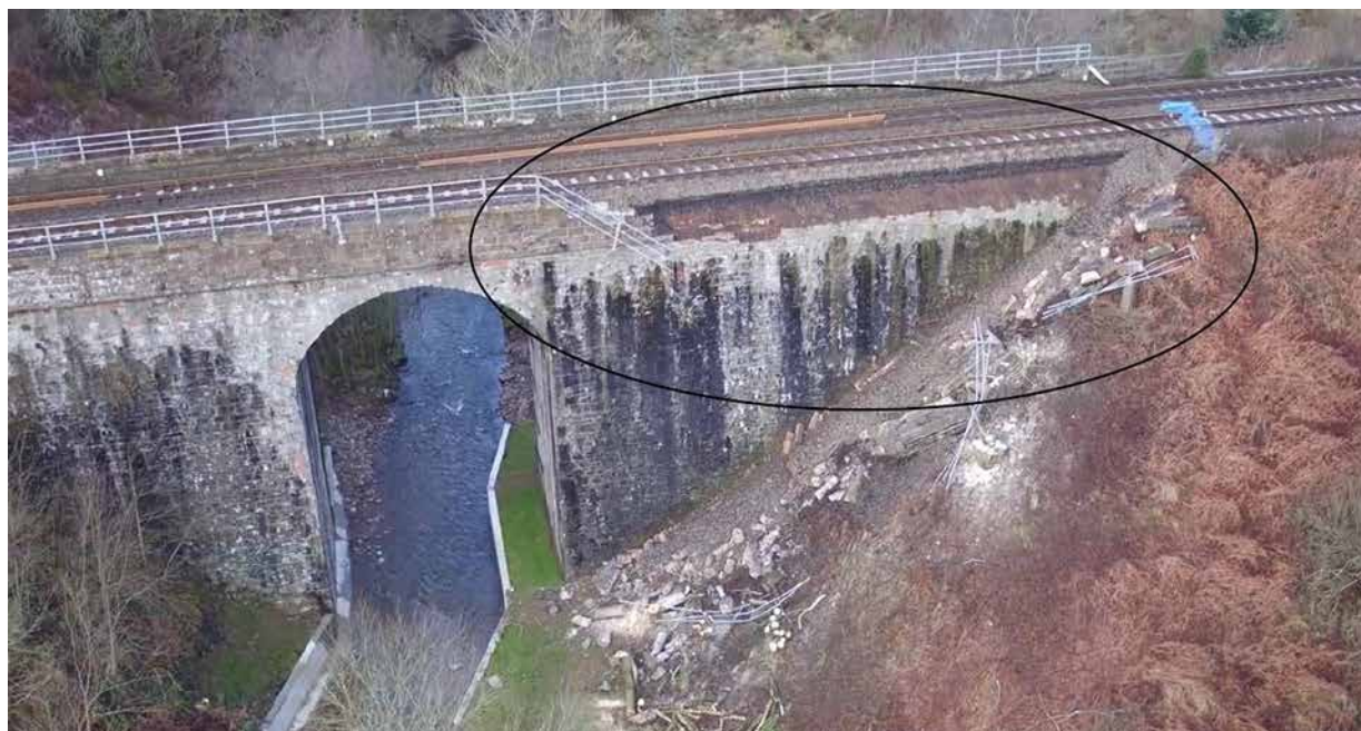
Figure M.1: South-east corner of bridge 328 following the failure of part of its parapet wall on 15 January 2021 (Network Rail)
