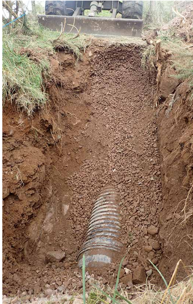
Figure 8: Gravel-filled drain close to washed out areas as exposed during post-accident excavations
