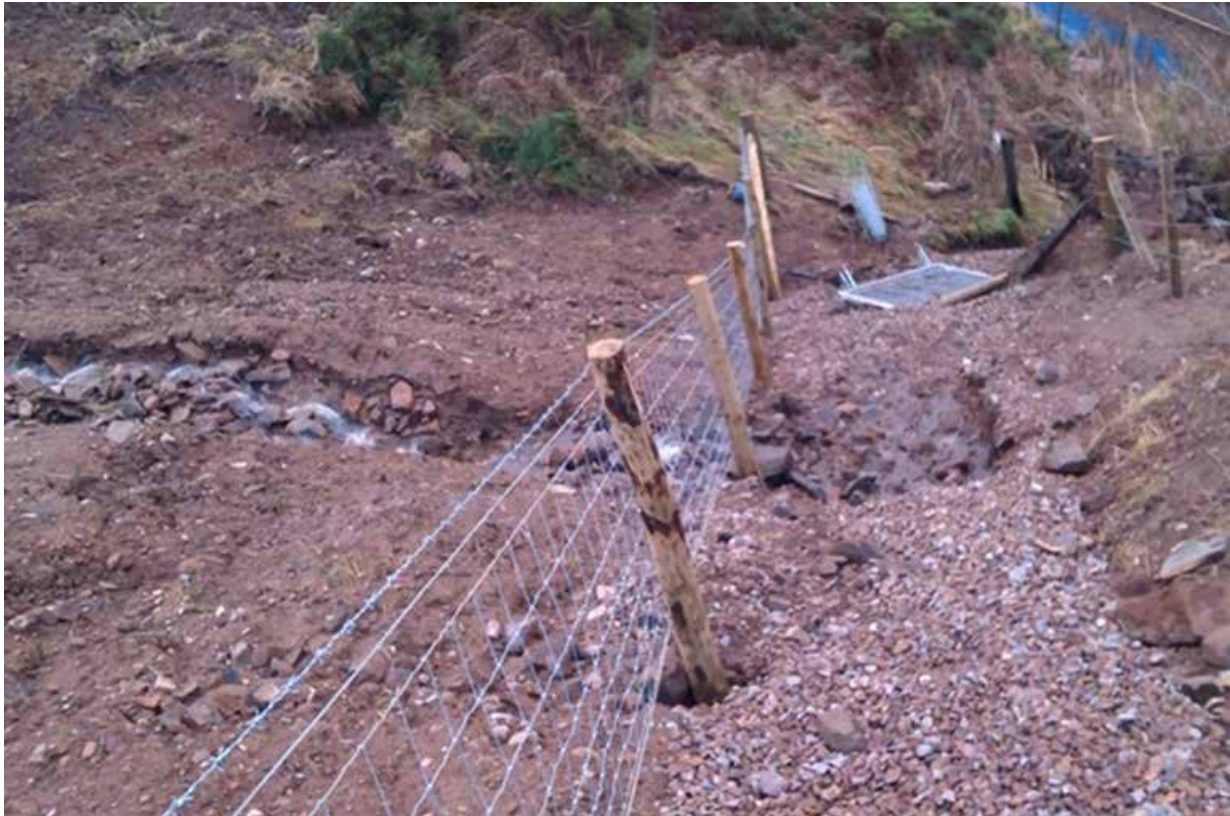
Figure 52: Surface of drain looking towards CP18 and railway in December 2012, before completion of the fencing (landowner)
