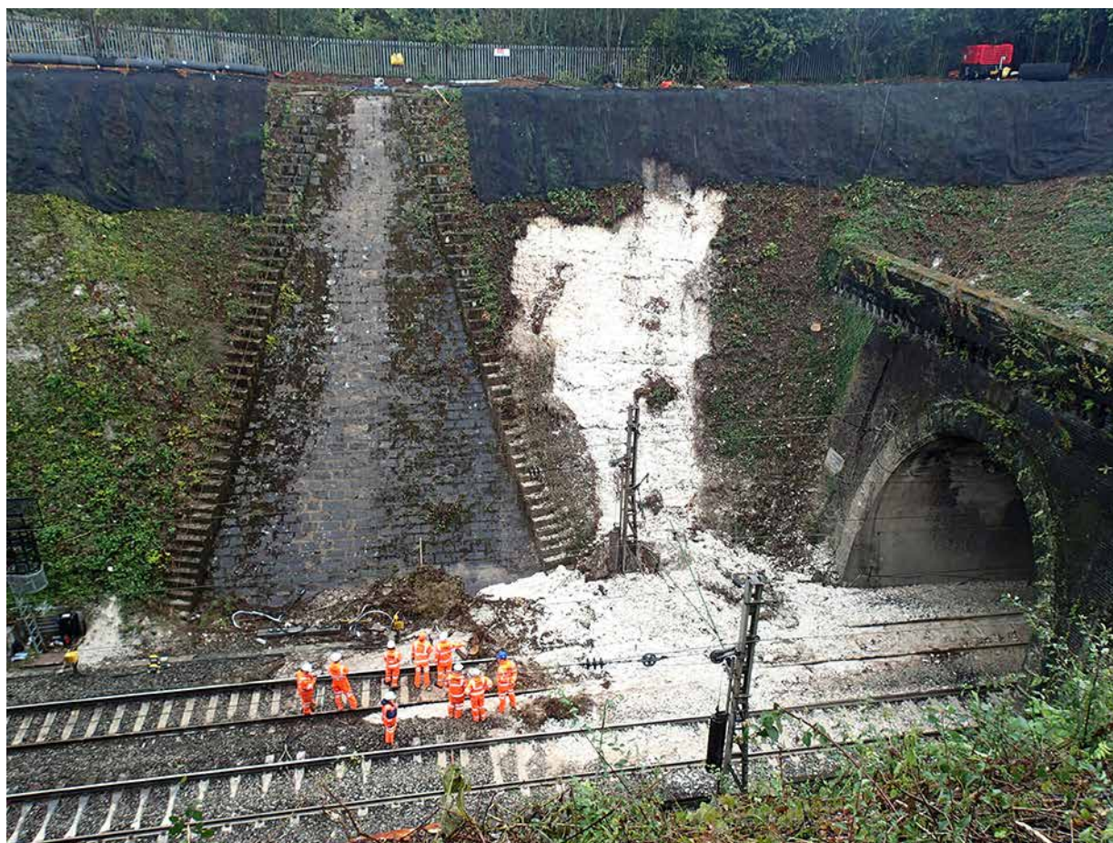
The landslip at Watford tunnel, September 2016
