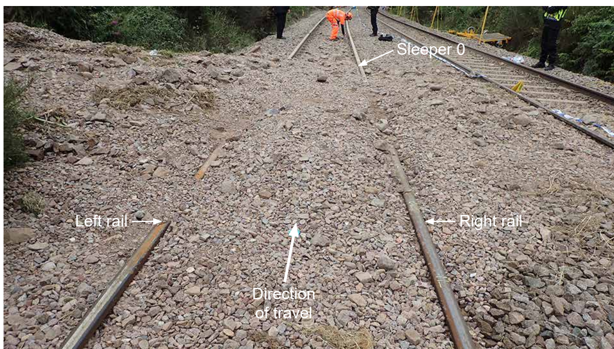
Washout debris covering the track
