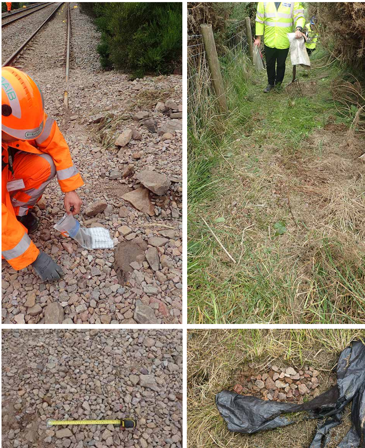
Figure 37: Landslip debris (left-hand images) and undamaged area of 2011/12 drain between washout and CP16. Surface of drain, probably protected by discarded plastic sheet since around the time it was constructed, shown in lower right image (Police Scotland)
