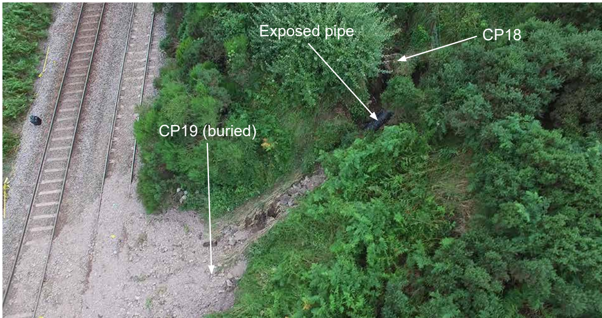
The washout (locations marked 'CP' are catchpits)
