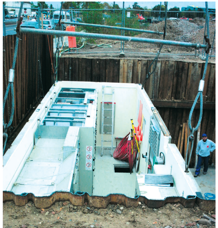
Saves space and is not visible: The traction power substation in the underground concrete container
