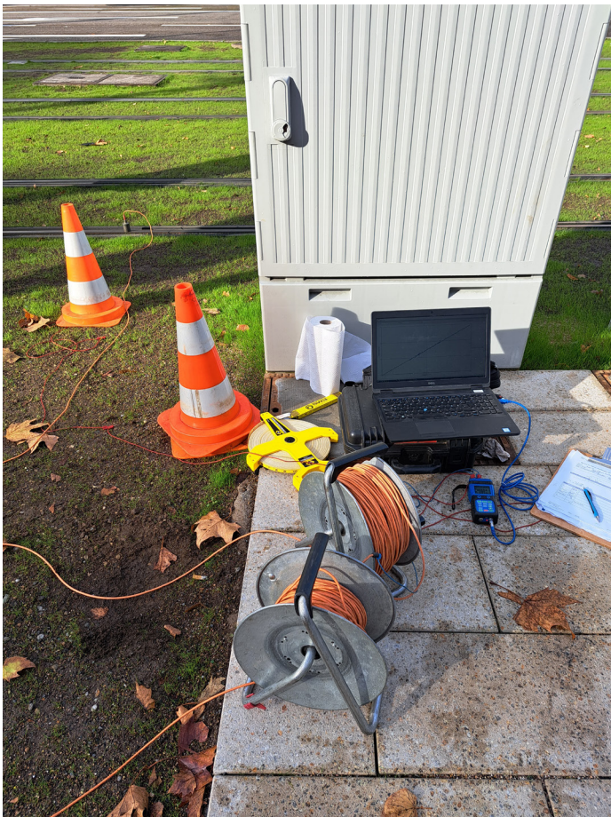
Measurements of leakage coatings
