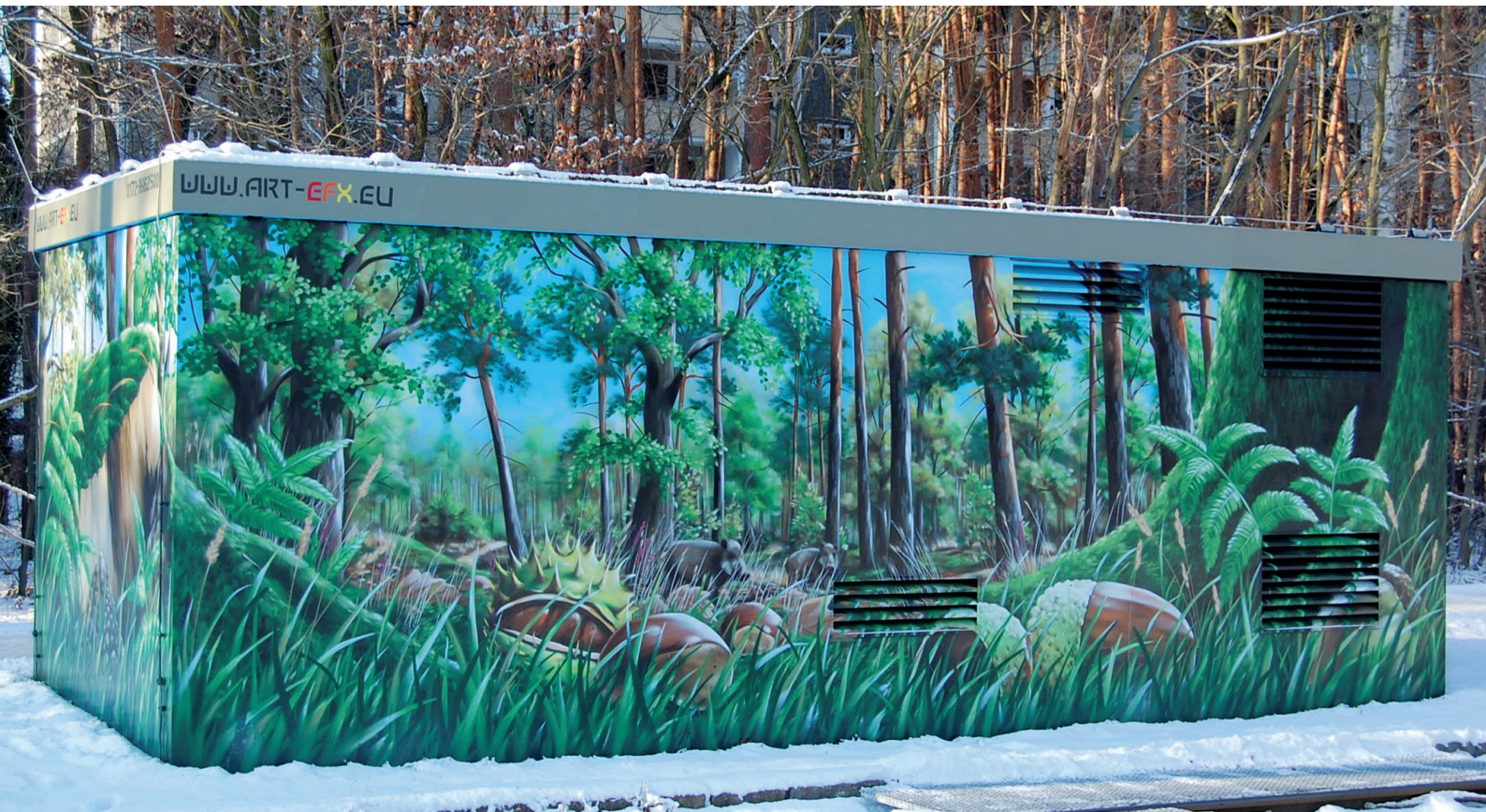
Substation in factory-made concrete container – e.g. for ViP Potsdam (DC 750 V)
