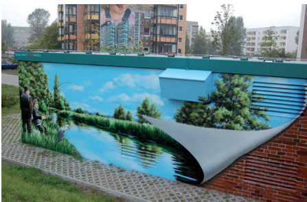
Turnkey substations – here for ViP Potsdam
