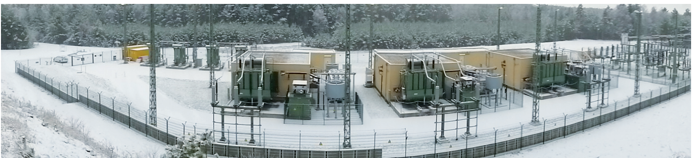
The inverter station of DB Energie Lohsa-West
